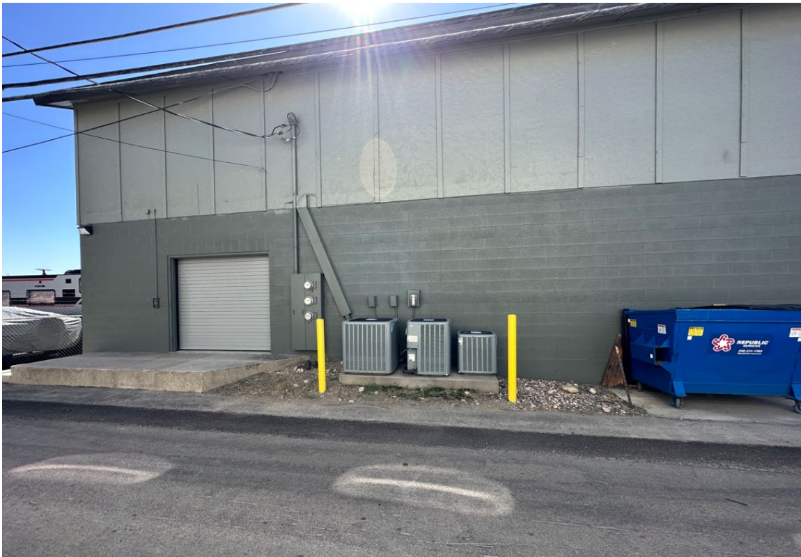
Figure 1: HVAC units and Trash Receptacle
